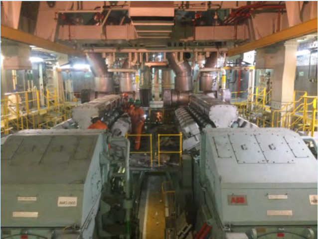
Efficient operation of well-maintained engines is critical to energy management.
